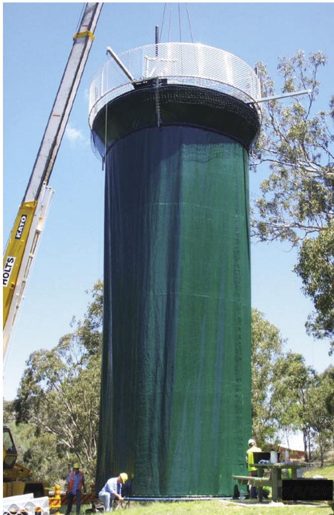
The reservoir mixer showing the extent of the collar which carries warm surface water towards the bottom of the reservoir
